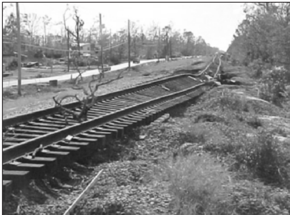
Katrina CSX Track damage in Waveland, MS.
