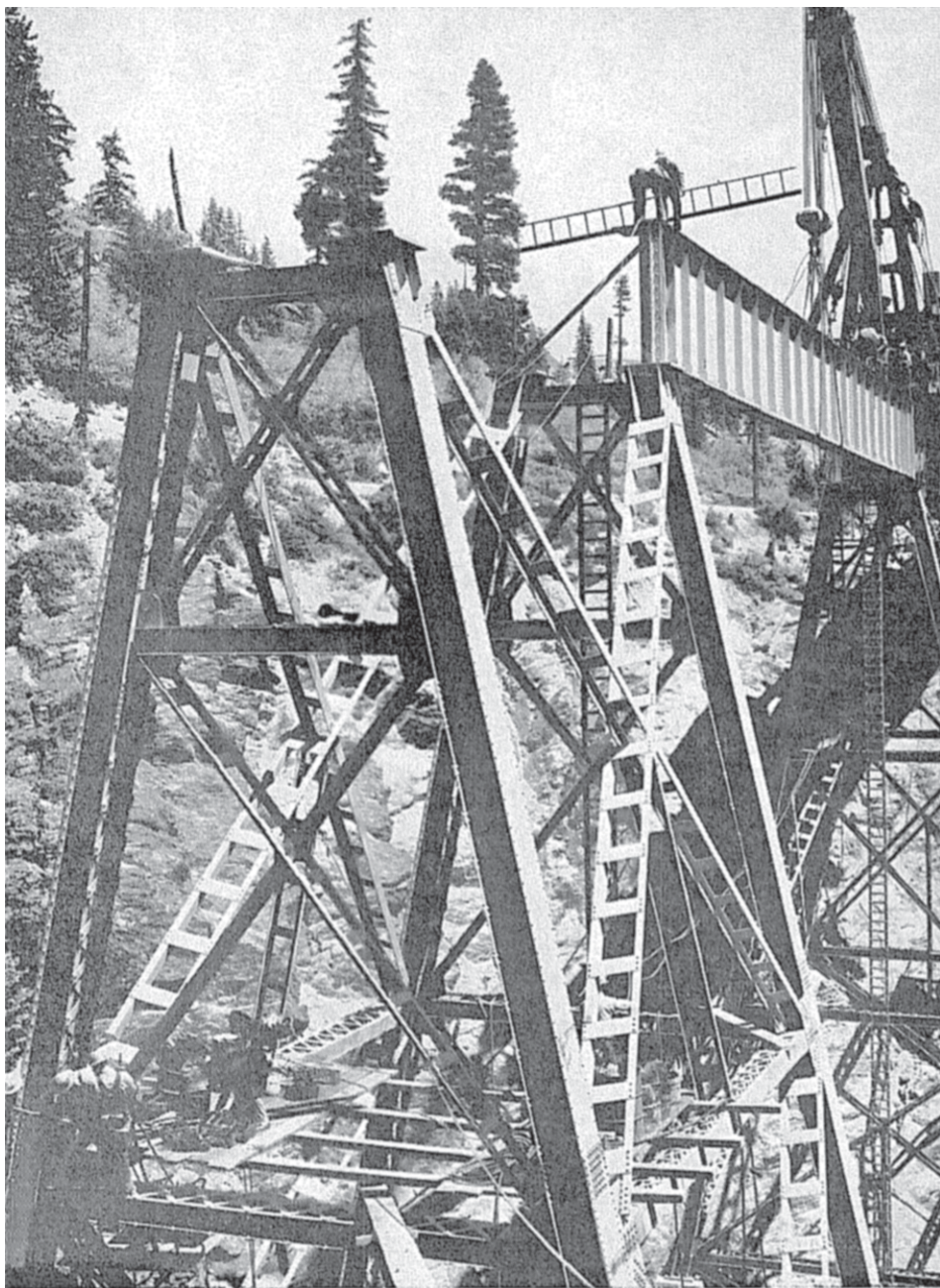
Above: A bridge under construction on the Great Northern Railway to be maintained by maintenance of way workers. The job of lowering the 37-ton girder took three and one-half hours.
