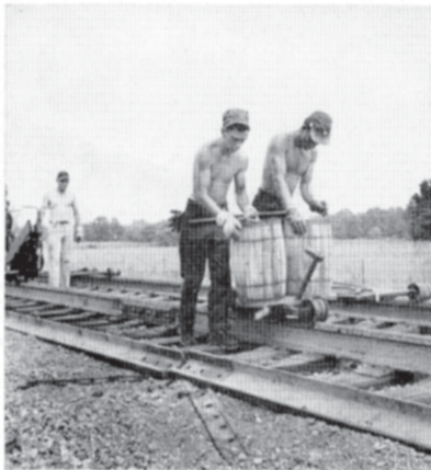
Above: To begin the modern motif, two workmen distribute spikes ahead of the spike driver.
